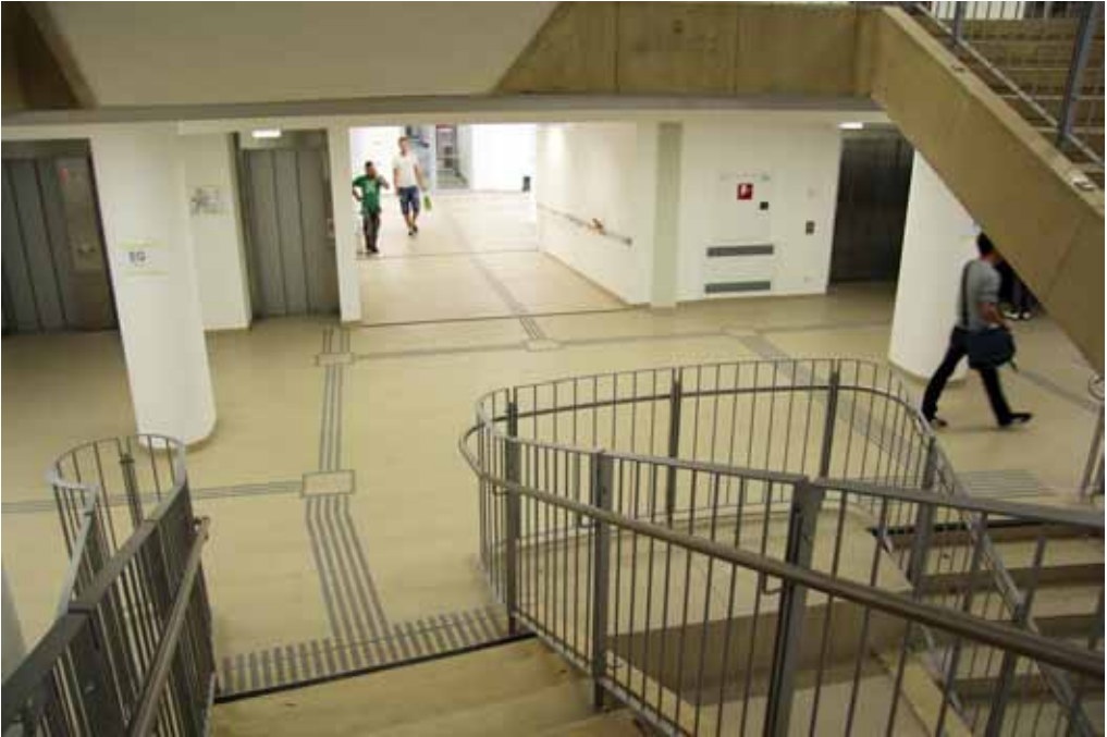
University of Vienna, Rossauer Lände 3, Austria. The polyurethane guiding system is arranged in accordance with the ISOTI standard. Self-adhesive strips are equipped with Gerband 941.
